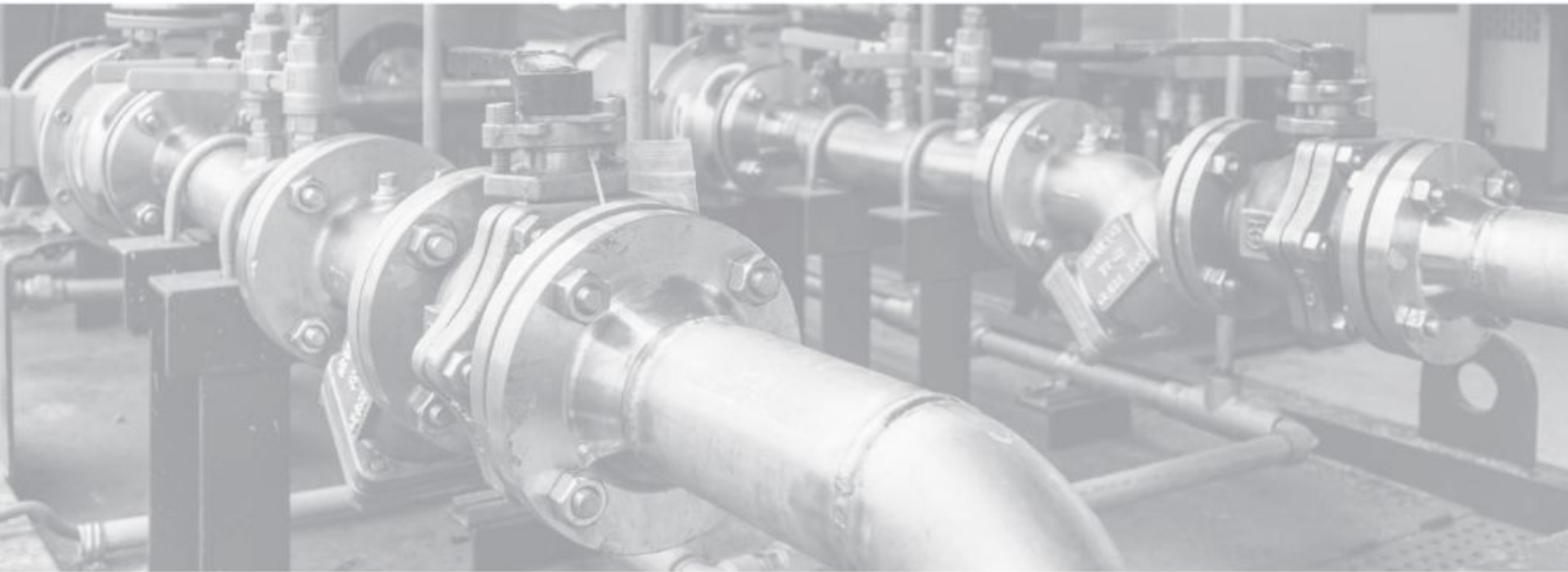
Light Industrial Park ,Ibn Rushed St - Yanbu KINGDOM OF SAUDI ARABIA
